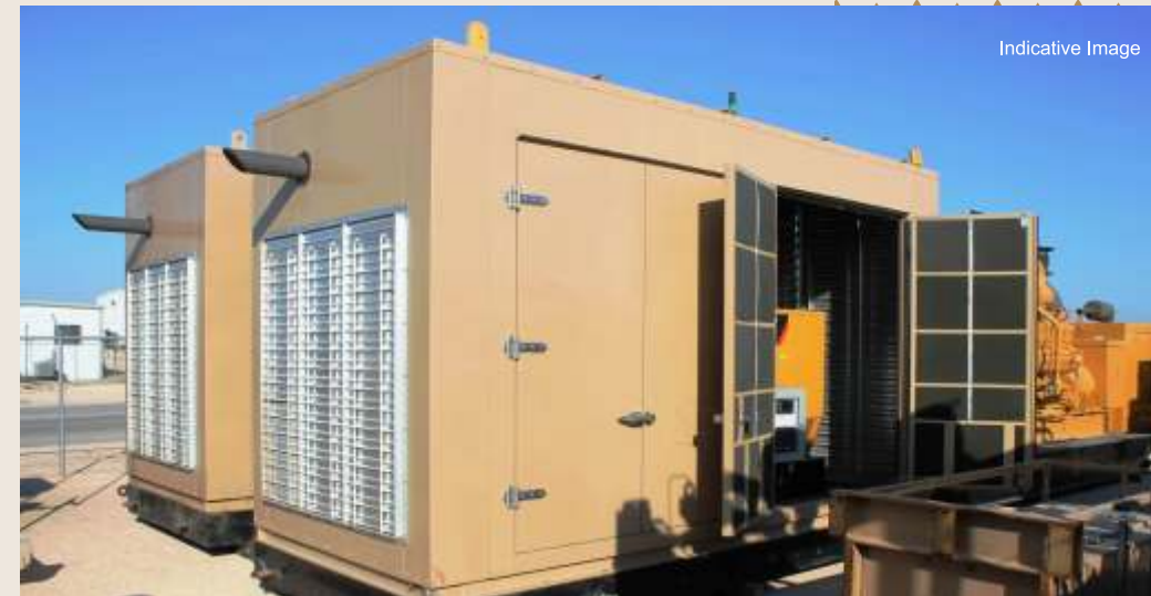
24 x 7 power backup
